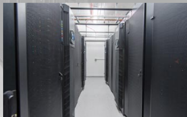
The SISSA/ICTP supercomputer Ulysses. The project was developed by SISSA through an agreement with ICTP, and the machine is housed in the "old" SISSA headquarters in via Beirut 2-4.
