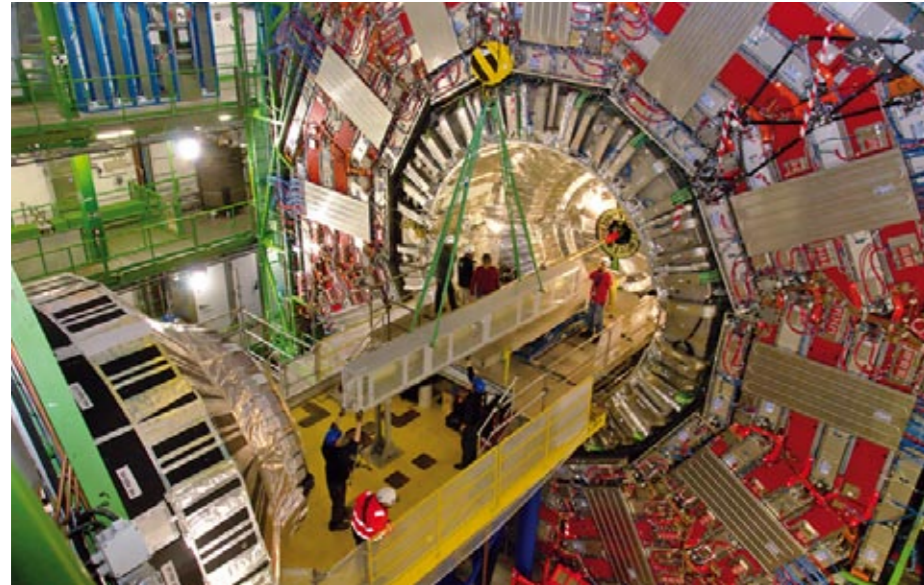
Installation of the CMS detector at the LHC experiment at CERN. Credits: CERN.
